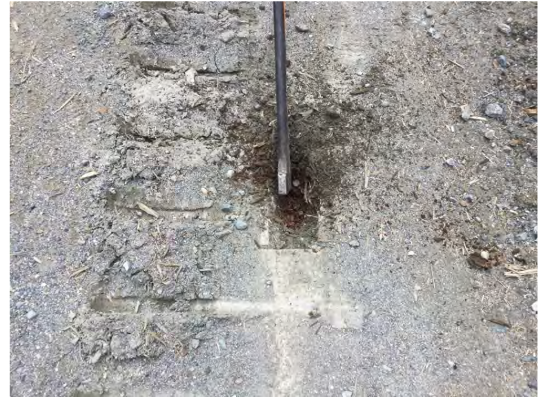
Timber plank condition (Poor) at Panel 2 wheel path - downstream left approach
