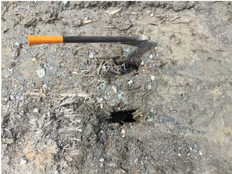
Timber plank condition (Poor) in Panel 7, downstream wheel path
