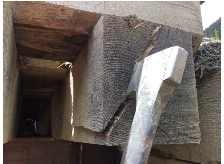
Panel 7 upstream cross-tie condition
