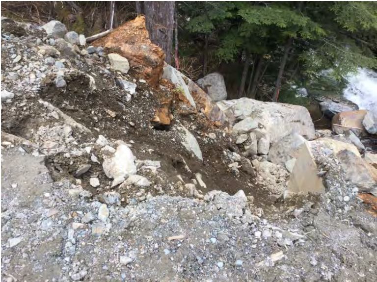
Fill slope has failed down stream left approach
