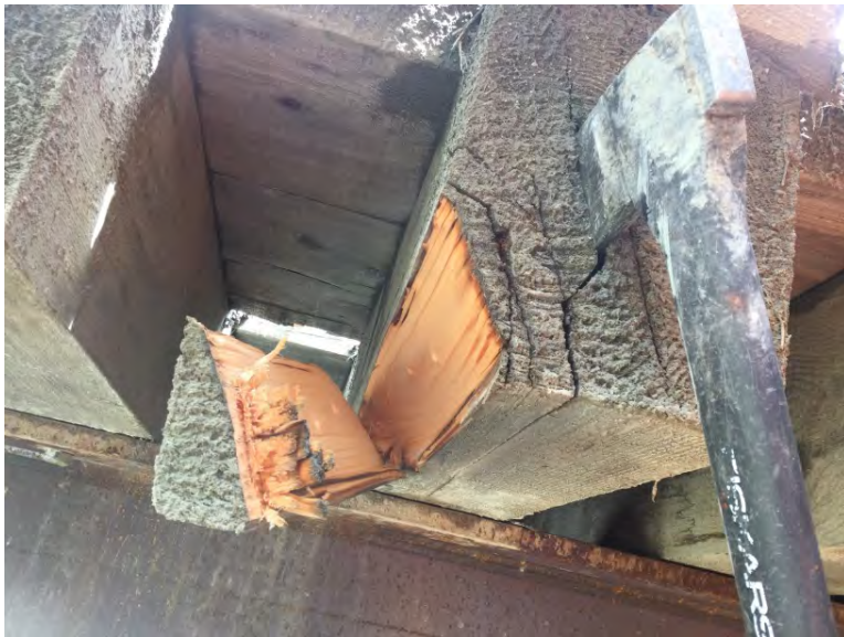
Panel 1 down stream cross-tie condition
