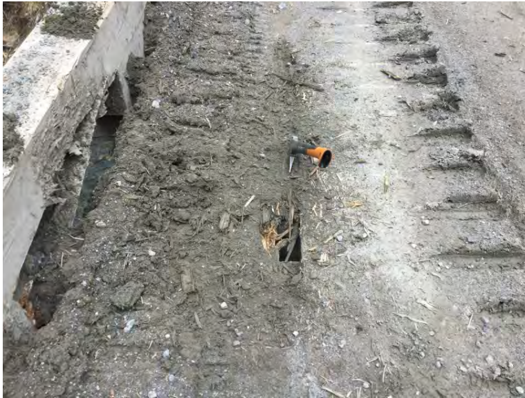
Hole in deck in Panel 1 at downstream left approach
